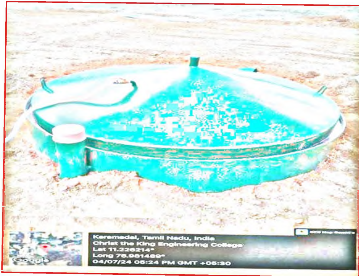
Bio-gas Plant installed inside Campus
